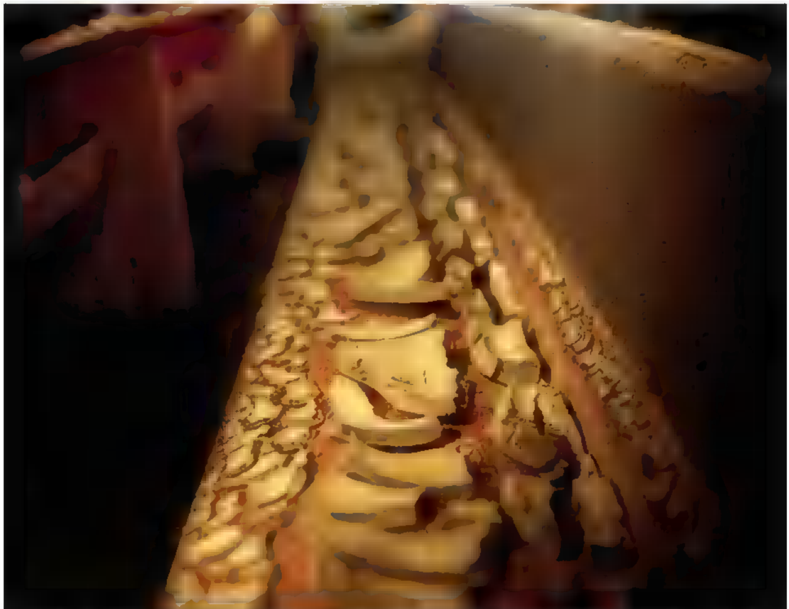
New Orleans Cracked mud upholsters the pews of the Greater St. Rose Baptist Church in the Lower Ninth Ward, where water rose more than 12 feet after the Industrial Canal levee failed.
